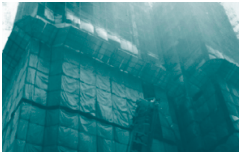
During the construction period, construction site should be covered up with dustcovers.
