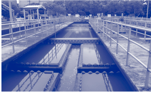
most companies have already installed wastewater treatment facilities
