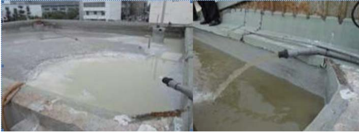
▶ Wastewater and sludge being stored illegally on a rooftop
