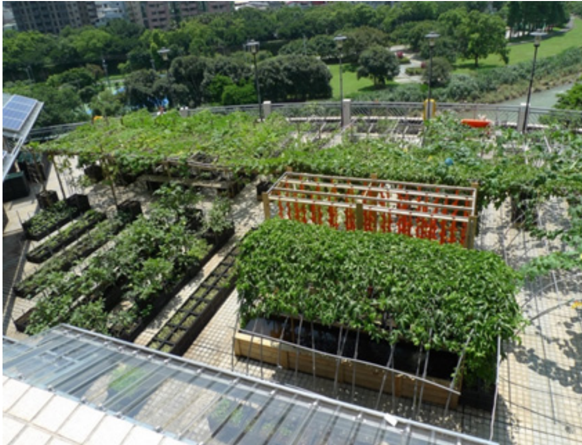
▲ Installing a green roof with solar power equipment to shade the building and cool down the temperature.
