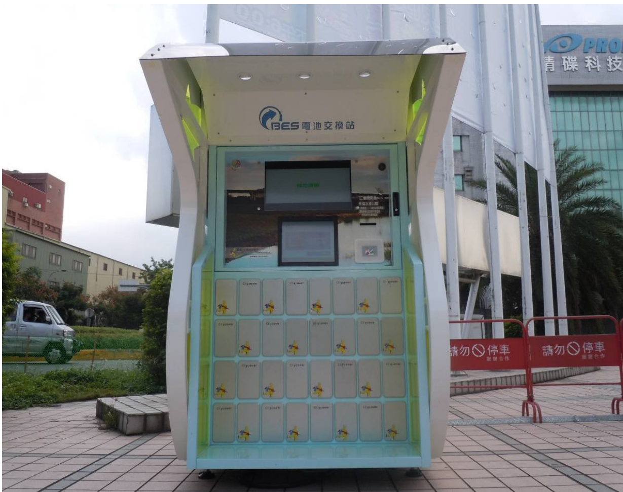
▶ Battery swapping station (photo: Citypower Taiwan Co. Ltd)
