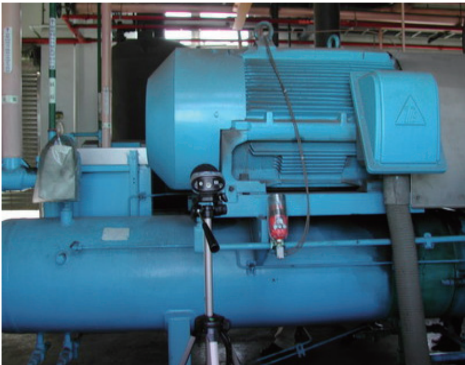
▶ Water pumps are often a source of low frequency noise
