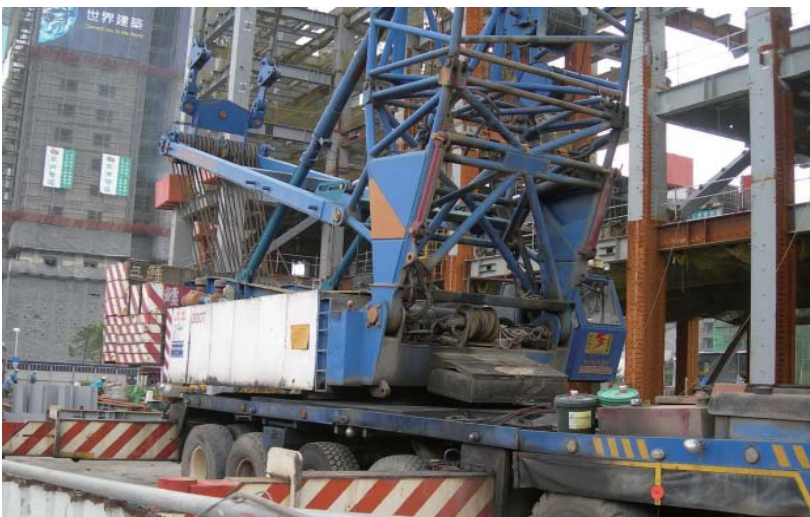
▶ EPA conducts random checks of petroleum products used in construction machinery at construction sites
