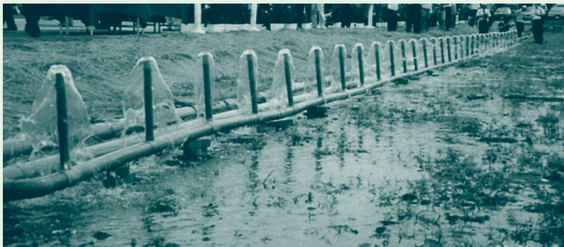
This is the first time constructed wetlands have been used to improve the quality of river water in Taiwan.
